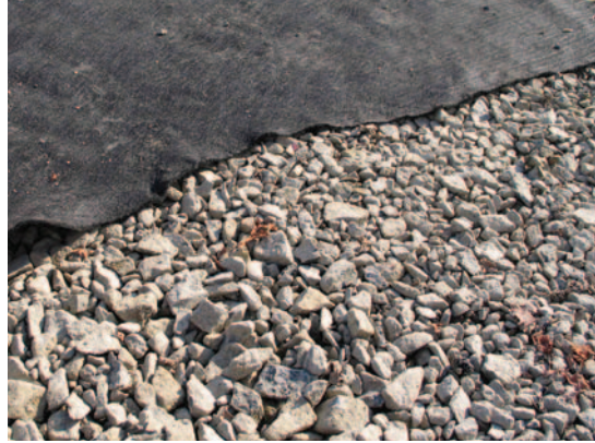
Figure 7. The drainage blanket of open-graded stone base ranged in size from 4 in. (100 mm) to 1/16 in. (2 mm), an Oregon DOT standard for large size, open-graded stone.
