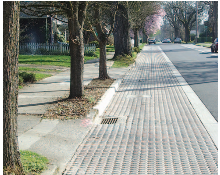
Figure 4. Deteriorated concrete curbs and driveway aprons were replaced. The existing storm drainage inlets and pipes were left in place for use as an overflow drain during heavy rainfall.
