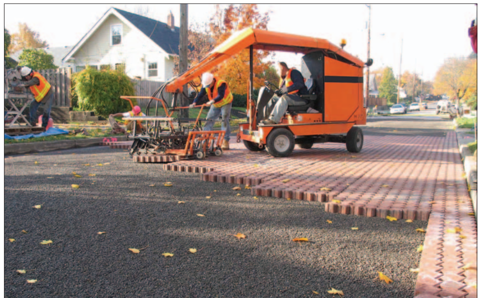
Figure 5. Mechanical installation equipment places the permeable pavers in the final laying pattern over the bedding course.
