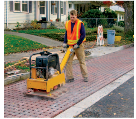
Figure 11. Installed pavers were compacted, the openings filled with the bedding stone and compacted to about 3/8 in. (10 mm) above the new concrete curbs.
