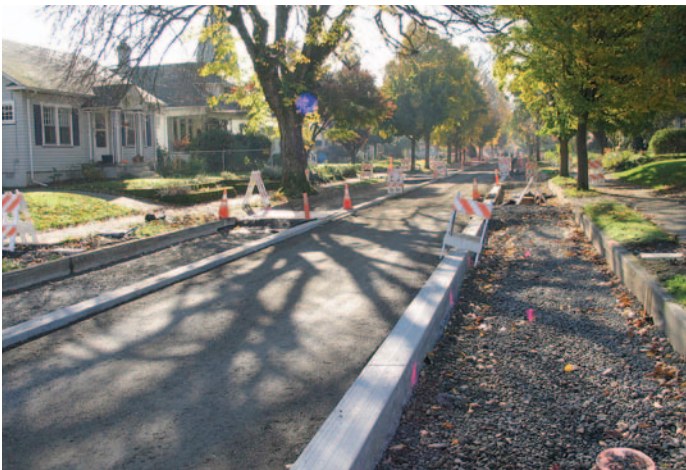
Figure 8. The drainage blanket base runs under the curbs across the width of the street. Geotextile was placed over the top of the drainage blanket in the asphalt center strip and dense-graded base compacted into place as shown here. Temporary driveways built with base and plywood allowed access to residents' driveways.
