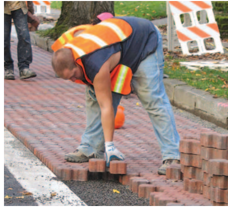
Figure 10. The width of new curb was set to accommodate mechanical placement of two paver layer widths within the 6 ft - 10 in. (2.1 m) wide parking strips. Some adjustments were necessary to fit the layers within the new curbs and the mostly uneven old curbs adjacent to the residences.
